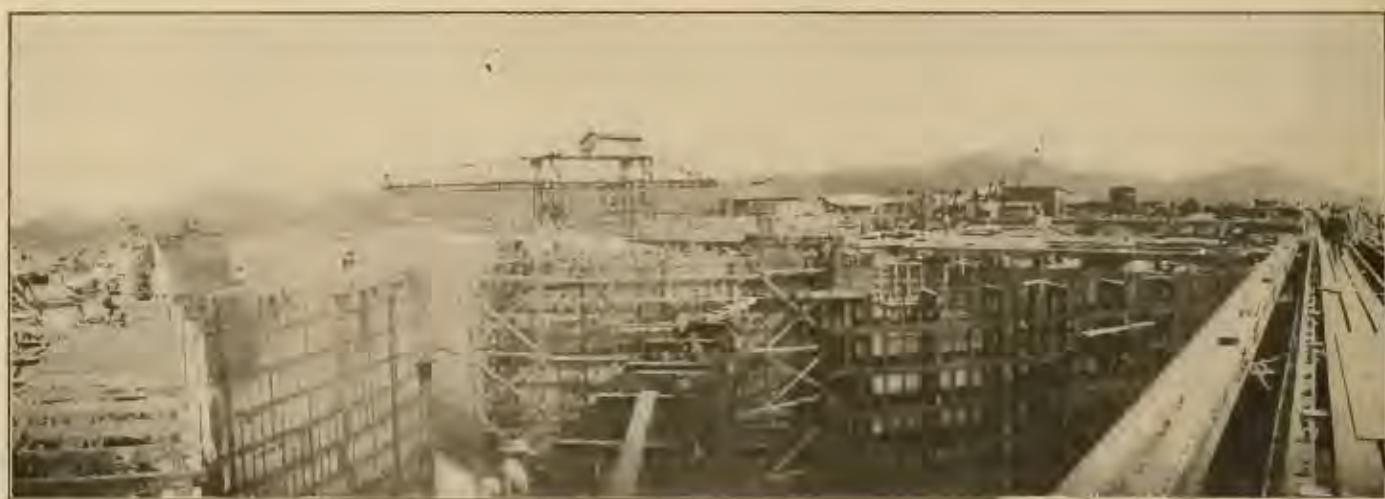
THE TANGLED MAZE OF STEEL SKELETONS THAT ARE A LOCK IN THE MAKING
